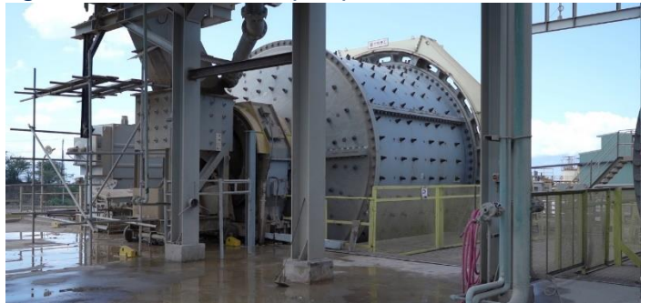
Figure 8. SAG Mill in Plant 2 (Palu)
